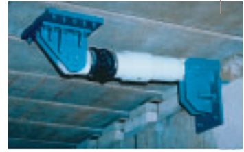
Placing on the pier head in the context of retrofitting (Hambrook bridge, UK)
